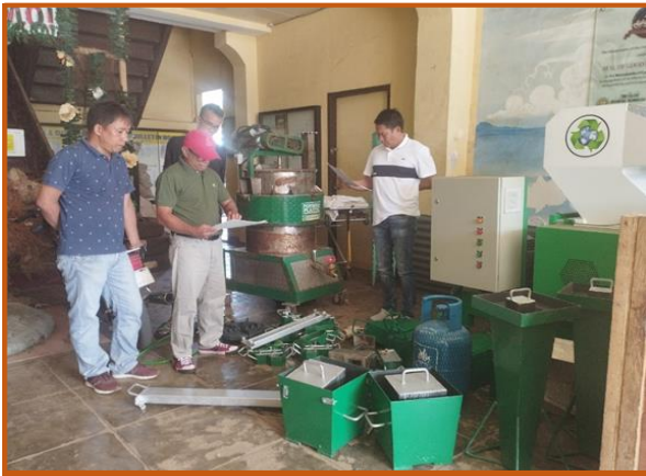
ASF Program Manager and Cuyo Chief Executive doing the inventory of Densifier Machine and other hardware before turn-over of the unit to the LGU.
